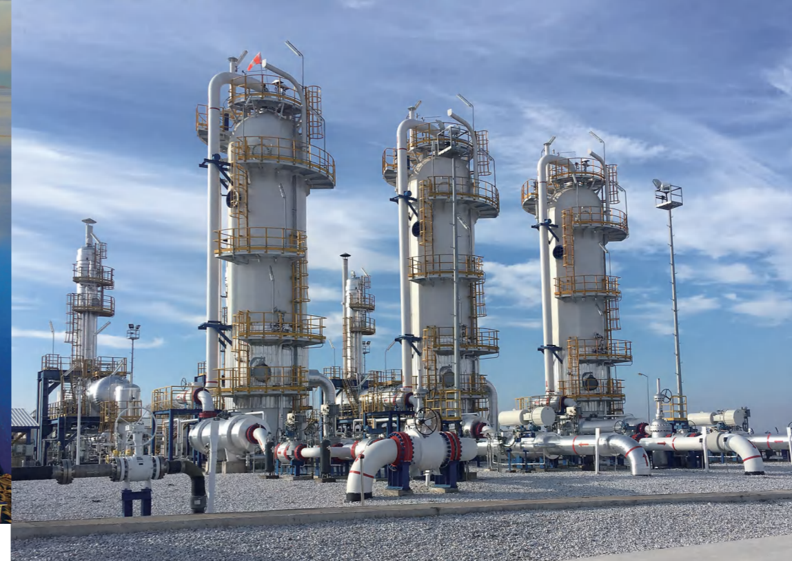
▲ Turkey Tuz Golu Underground Gas Storage Expansion Plant (storage capacity: 4 billion cubic meter, daily withdraw capacity: 40 million cubic meter, daily injection capacity: 30million cubic meter)
