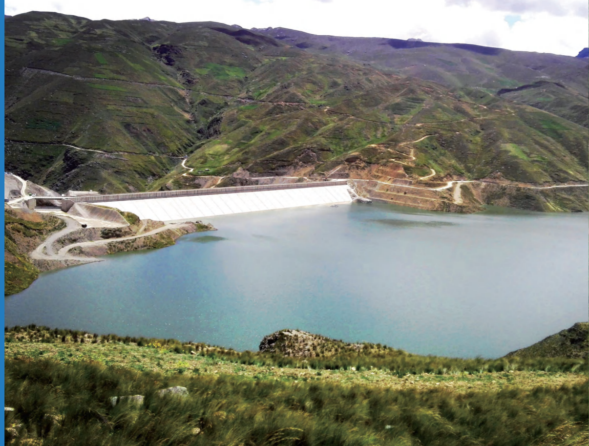
▲ Construction of the Misticuni Dam in Bolivia and ancillary works (altitude 3,700m, storage capacity of 150 million cubic meters)
