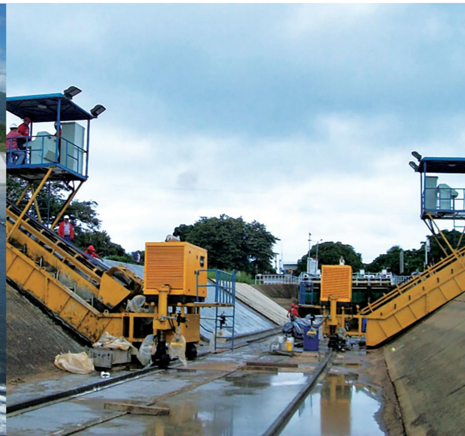
▼ Main Canal Construction in the Guarico Irrigation System Rehabilitation and Construction Project in Venezuela
