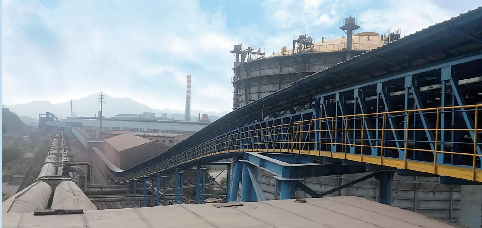
▲ Pipe Belt Conveyor System of Benxi Iron and Steel Group Company, Liaoning Province
