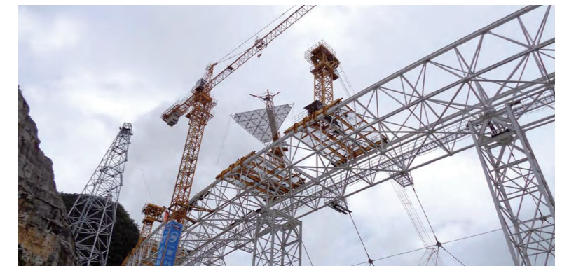
▲ Lifting of Reflecting Surface System for the Five-hundred-meter Aperture Spherical Radio Telescope (FAST)
