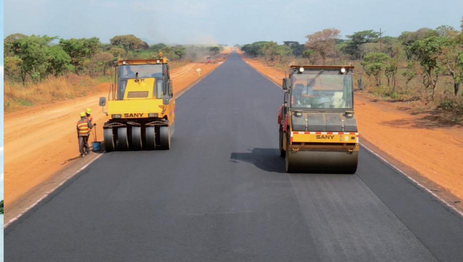
▲ Upgrading of Mbala - Nakonde (D1) Road (171.9km) in the Northern Province in Zambia (171.9km)
