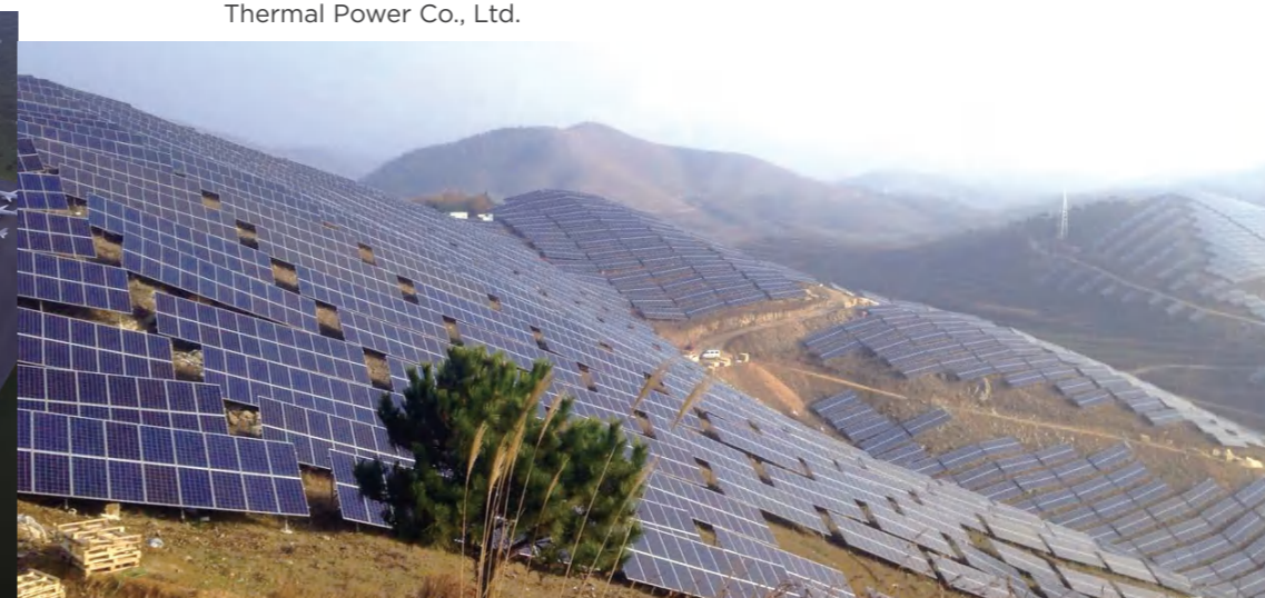
▲ 40MWp Photovoltaic Grid-connected Power Generation Project in Haiyang, Shandong
