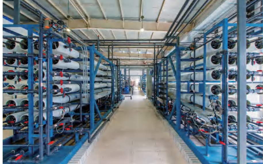
▲ Yangmei Taihua industrial wastewater treatment system in Taiyuan, Shan'xi Province
